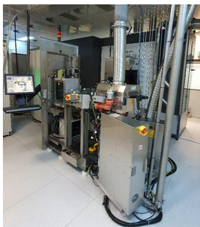
Overall View and User Control Interface
