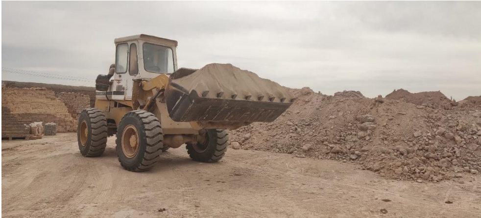
Figure 4.1. Loader machine with the ability to carry 2.5 tons inside the site to move soil
