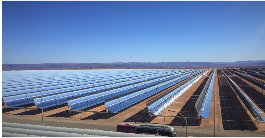
Figure 1.8: Parabolic trough collector field at the Ouarzazate Solar Power Station Project – Phase I, also known as Noor I [25].
